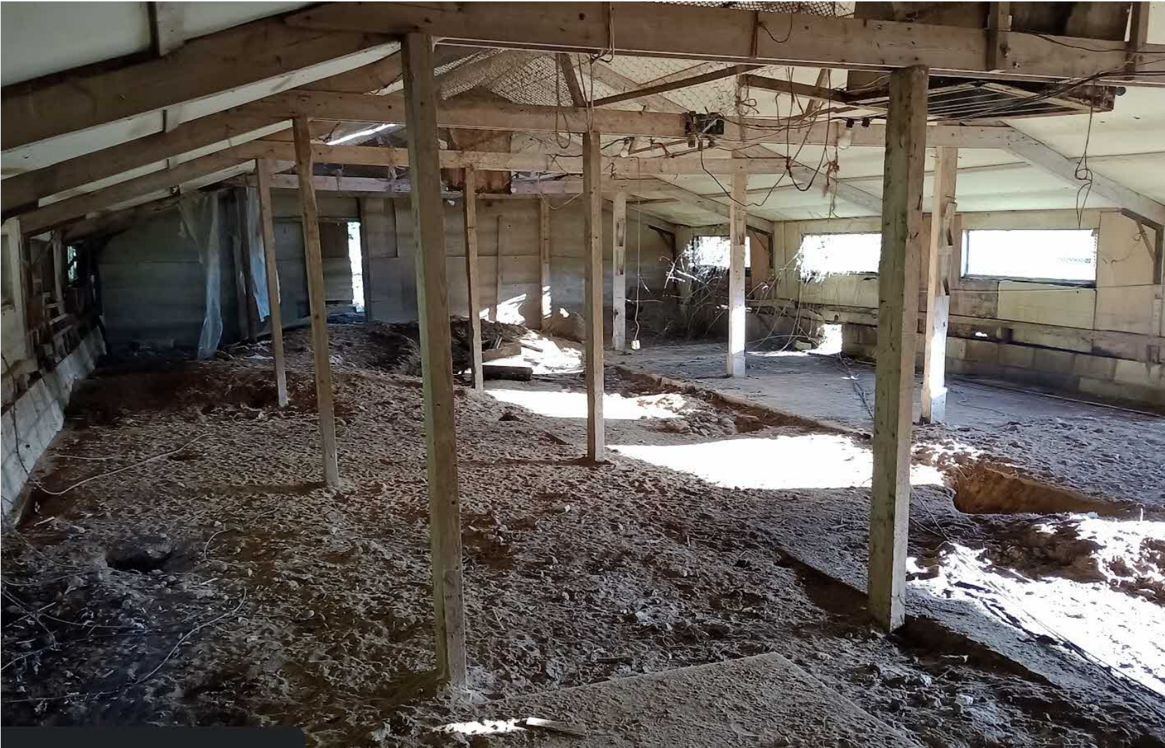
Internal view of barn showing roof trusses and internal floor slabs and posts
