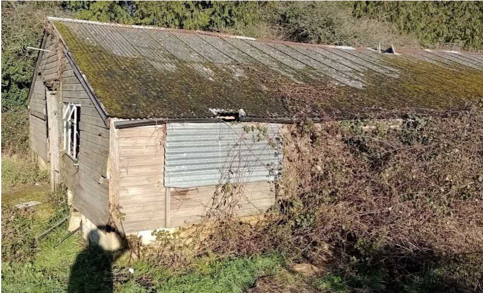
External blockwork lower walls and timebr clad timber external walls and metal sheeting roof (Front and side wall)
