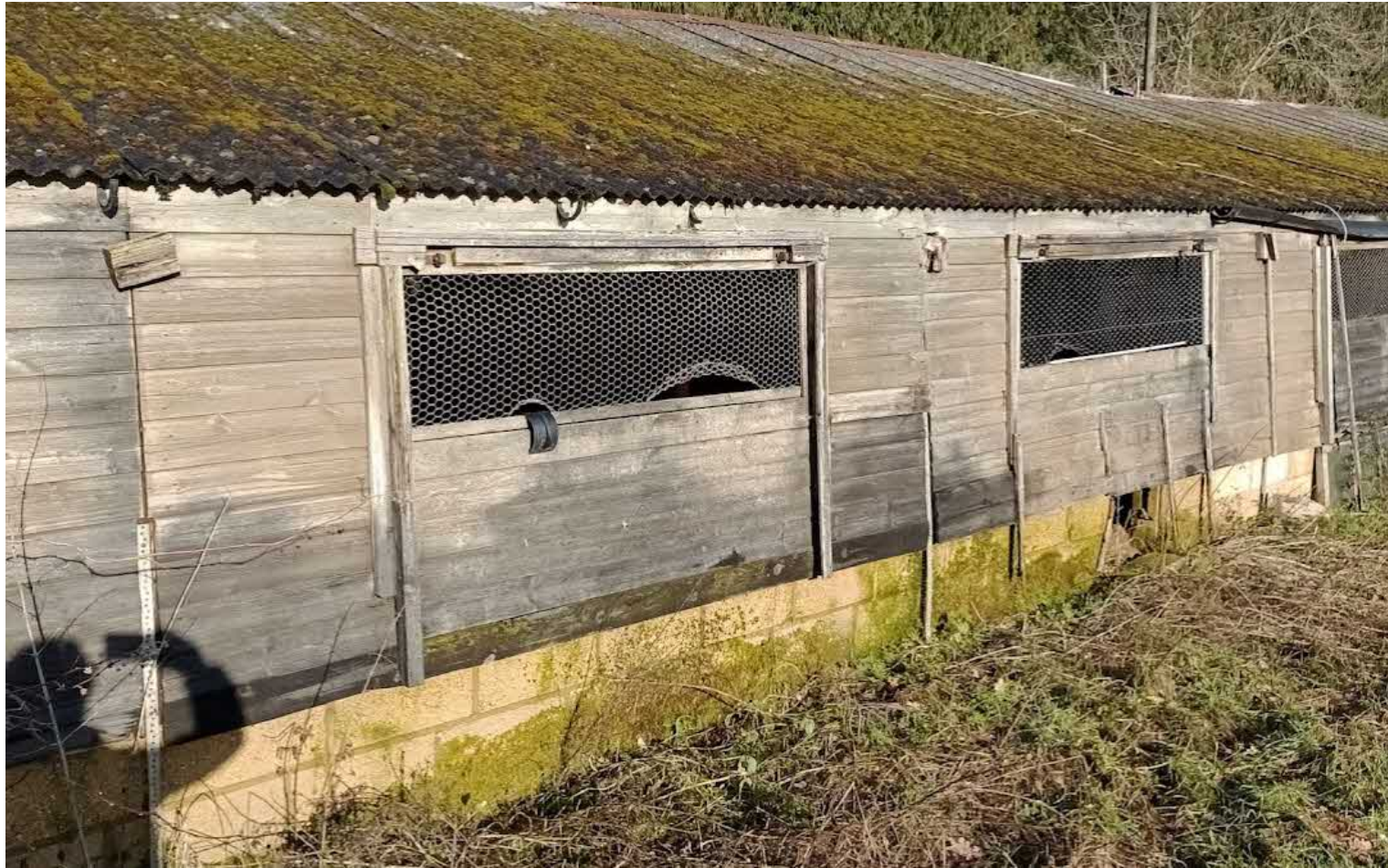
External blockwork lower walls and timebr clad timber external walls and metal sheeting roof (Side wall)
