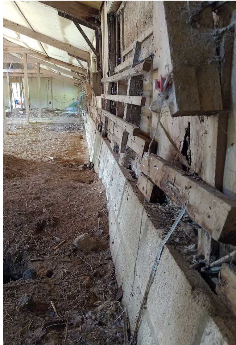
Leaning side wall needs to be re-built
